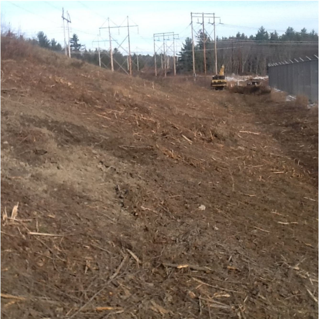
Photo #11 , Deerfield substation 2016.
