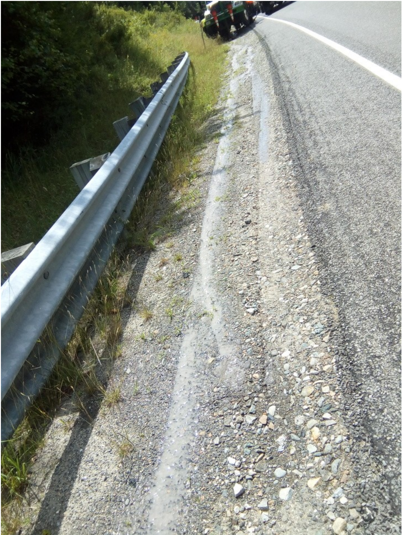
Photo #7 Slurry tub overflow draining down Route 112, WMNF
